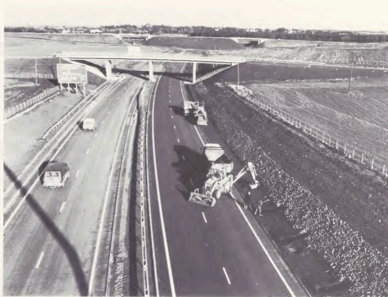
Monkton Lodge Access Overbridge with the Old Craighall Junction in the background
